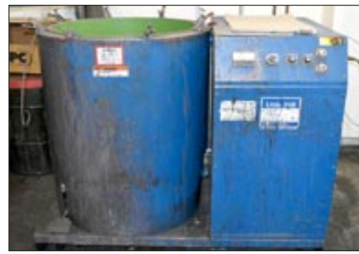
LITTLE STILL SOLVENT RECOVERY SYSTEM, WITH CHILLER
