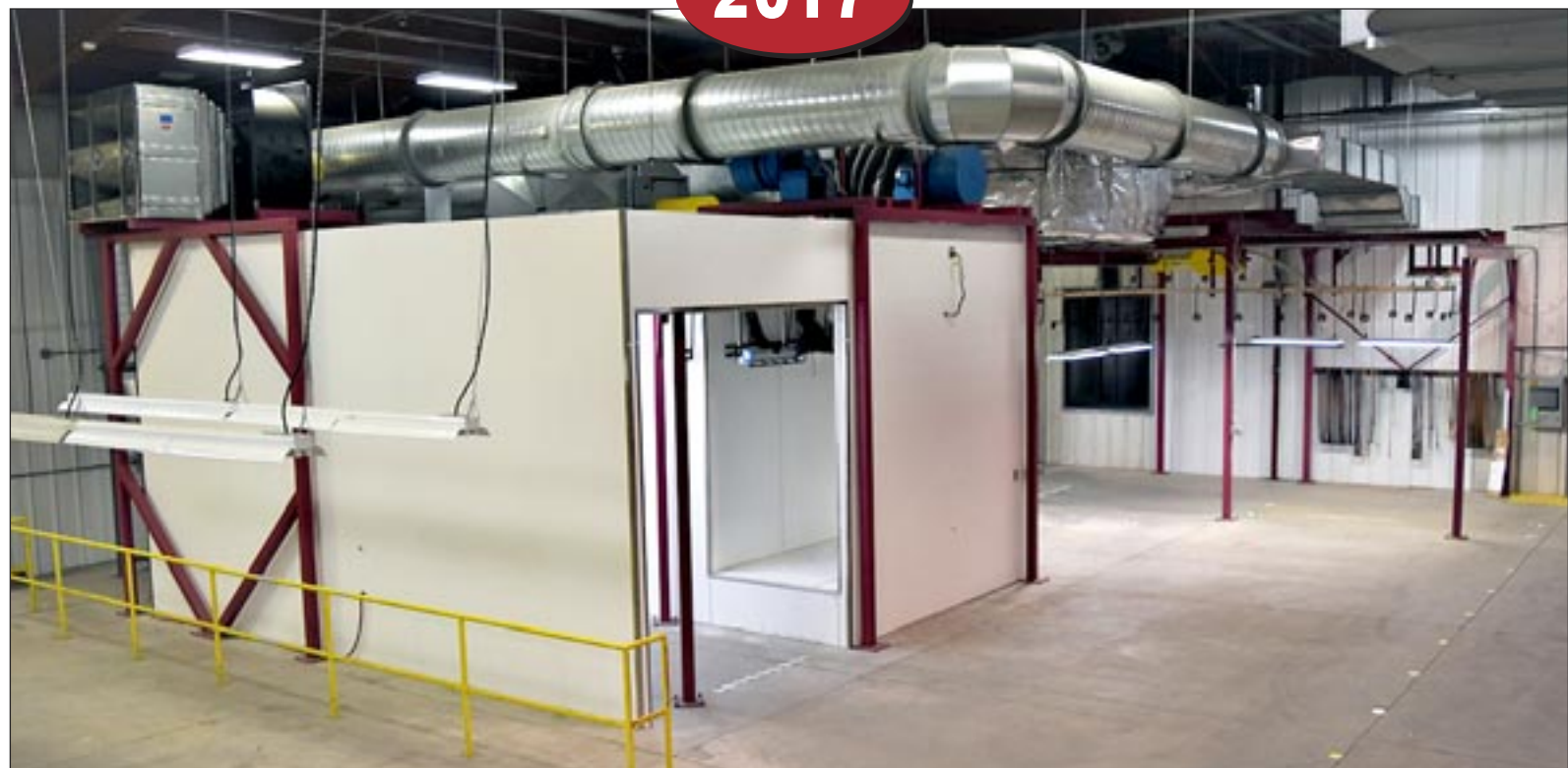
EXTERIOR VIEWS OF 2017 GLOBAL FINISHING SOLUTIONS ENTIRE CONTINUOUS PAINT SYSTEM
