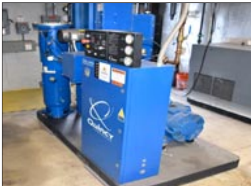
QUINCY 50-HP QSI-45I ROTARY SCREW AIR COMPRESSOR
