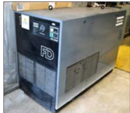
ATLAS COPCO FD345 AIR DRYER
